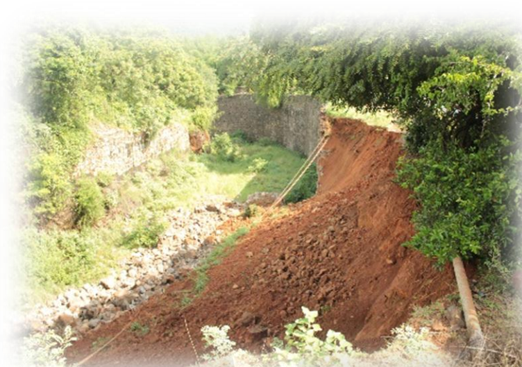
COLLAPSED WALL OF THE TIGER ENCLOSURE
